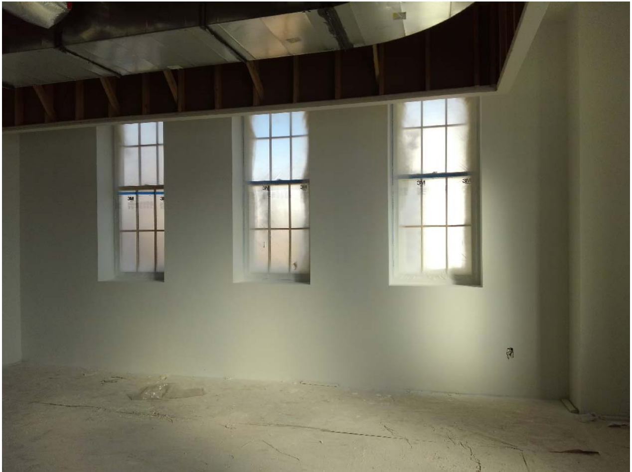
Painting continues on the third floor. Classrooms getting more coats of paint...
