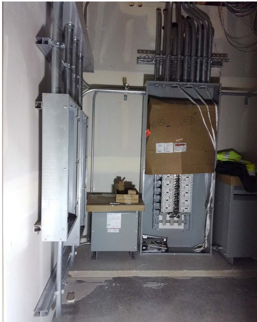
The 1 st floor electrical sub-panels...these will be powered up on the weekend of Dec. 16 th & 17 th .
