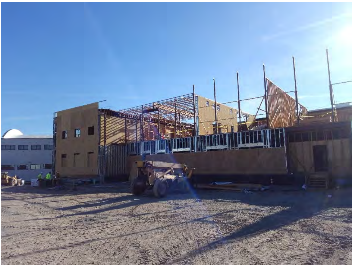
Installing the West and East wing ceiling joists and roof sheeting... This will help the crew when they set the trusses.
