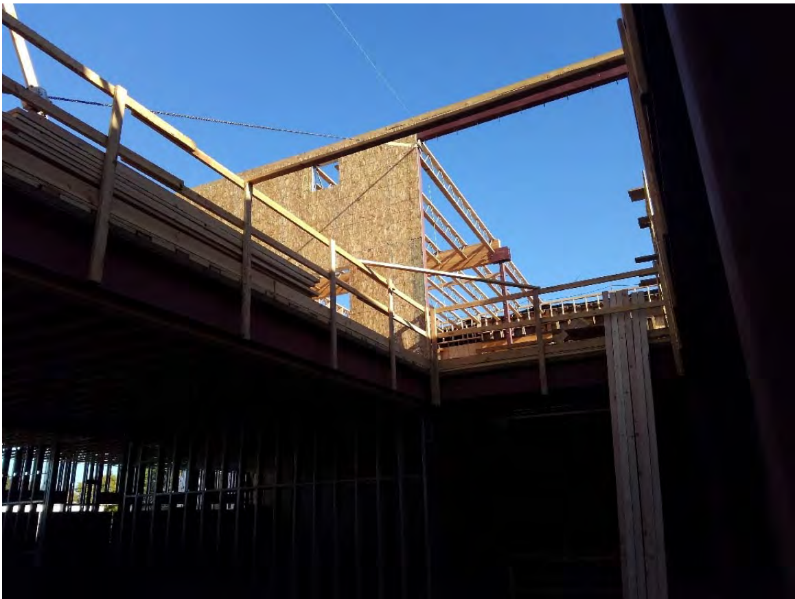
2 nd Floor walls going up around the front office area (top), and a view up the stairwell ( 2 nd floor landing).
