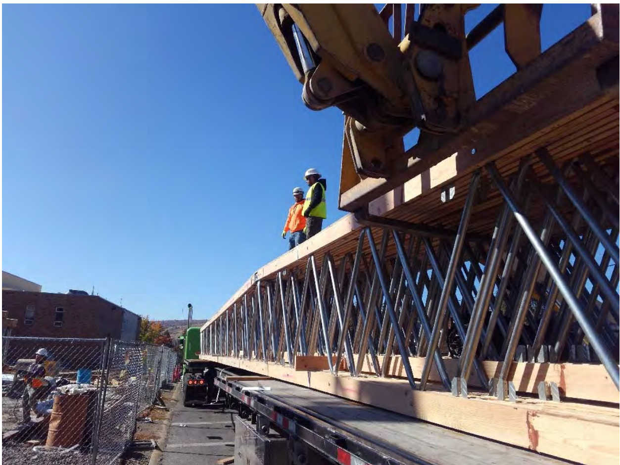
Preparing to unload the Roof Trusses for the 3 rd floor Media Center.
