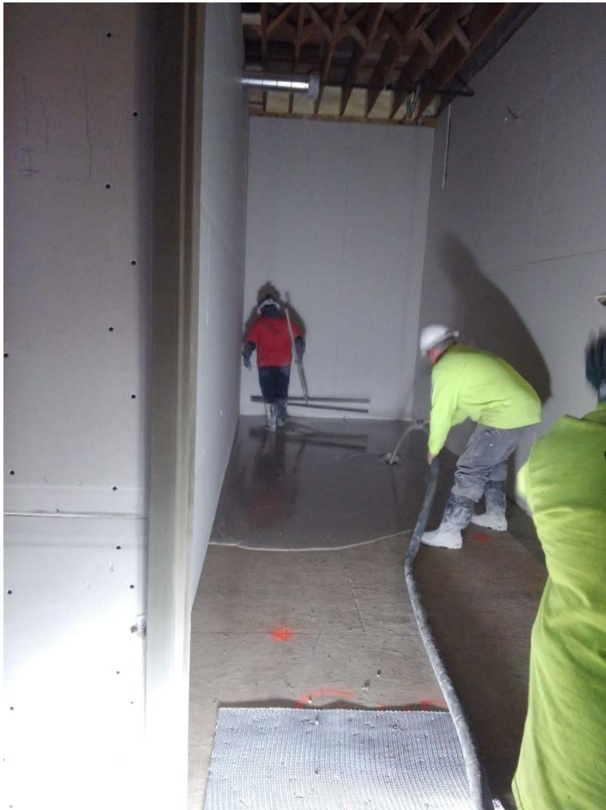
A storage room...you can see the markers which help the installers get the correct thickness.
