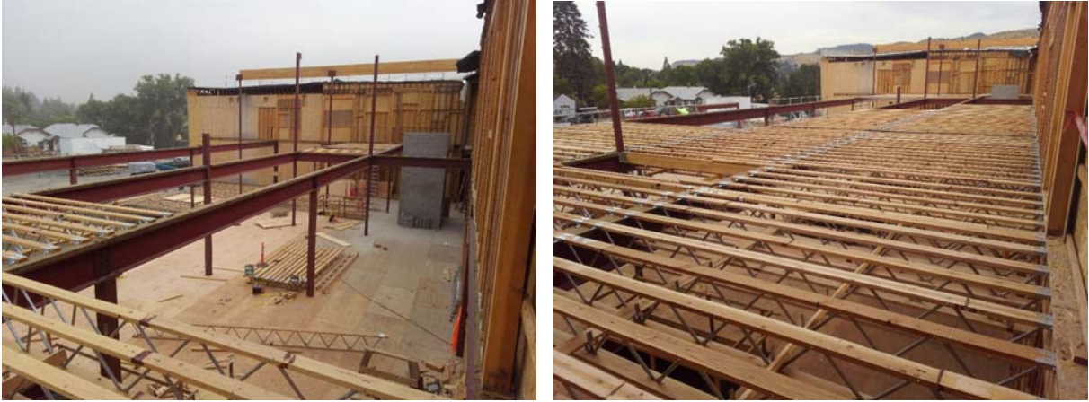
Floor Joists on the Third Floor. Last week (left side), compared to this week (right side).
